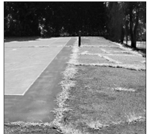
5th Avenue tennis court is in unplayable condition. City has budgeted cash to begin repairs. File photo.
